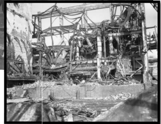
Detail of the damage.
